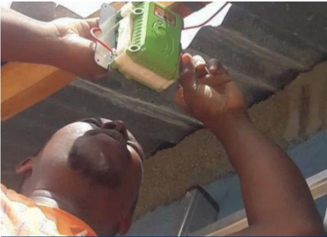
A sensor is installed at a borehole well site
